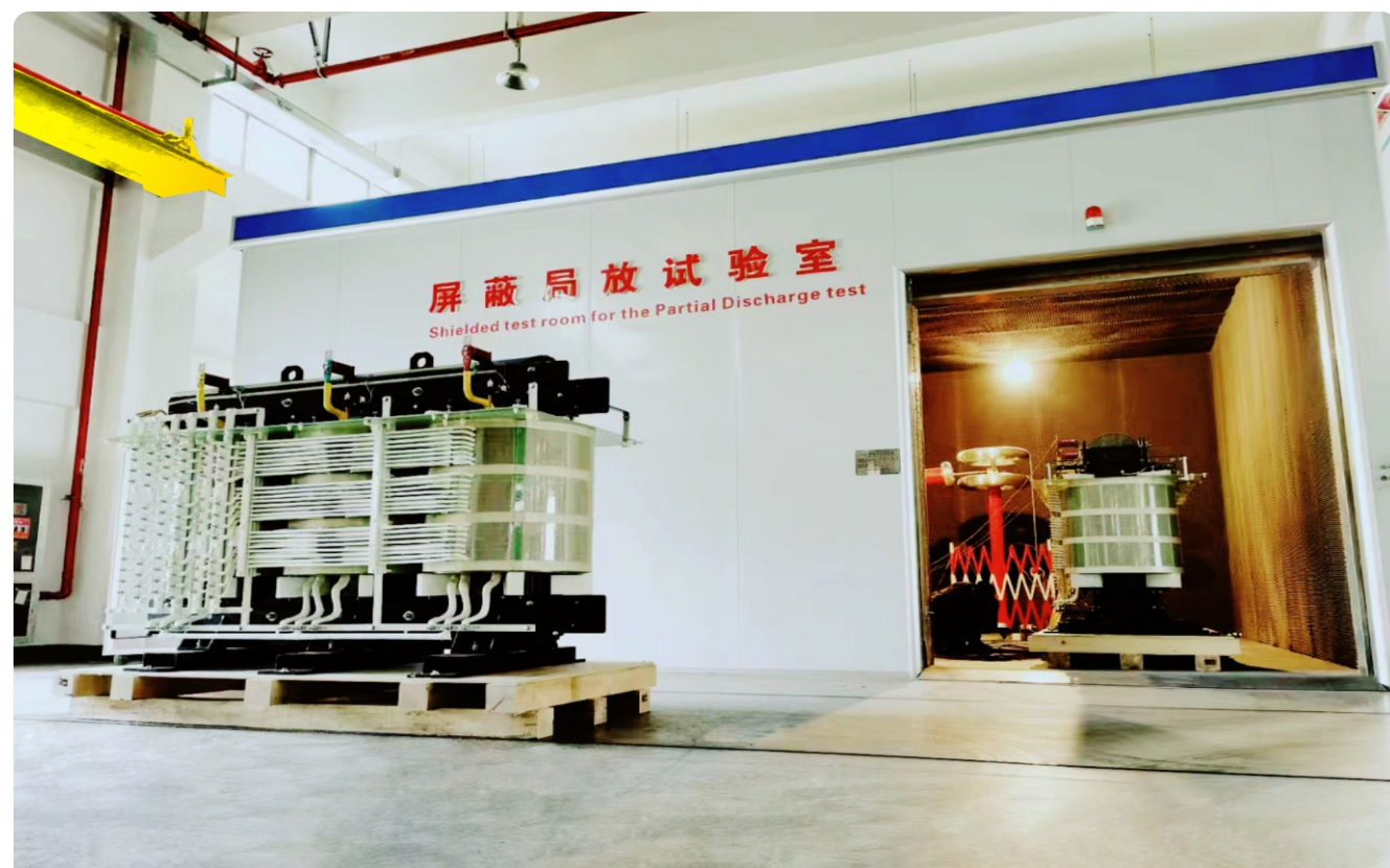
Partial discharge testing equipment min 1pc background PD
