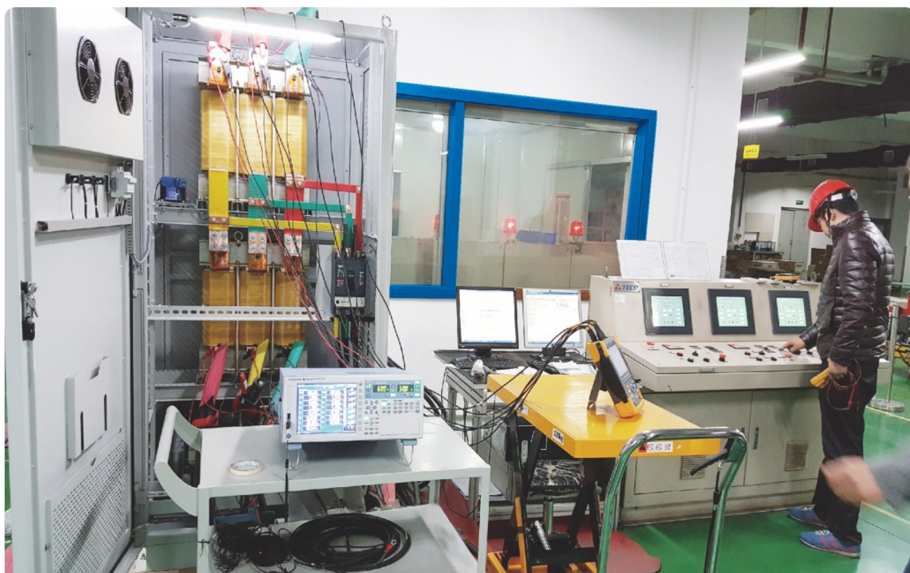
Passive harmonic filter performance testing
