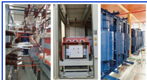
34.5KV 6 taps reactors ABB (Canada) project
