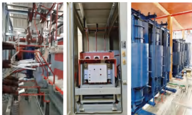
34.5KV 6 taps reactors Metal Refining project ABB (Canada)
