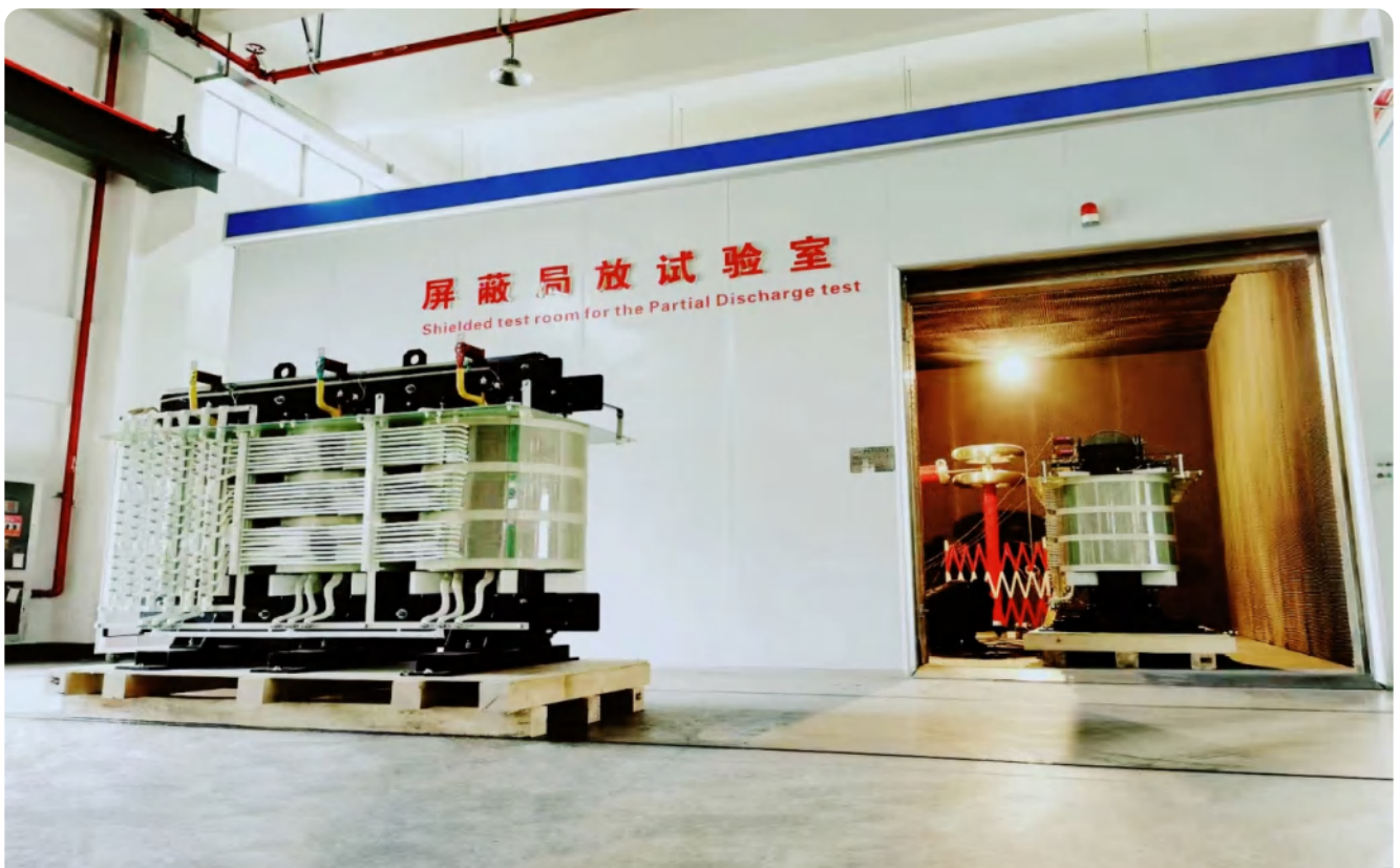
Partial discharge testing equipment min 1pc background PD
