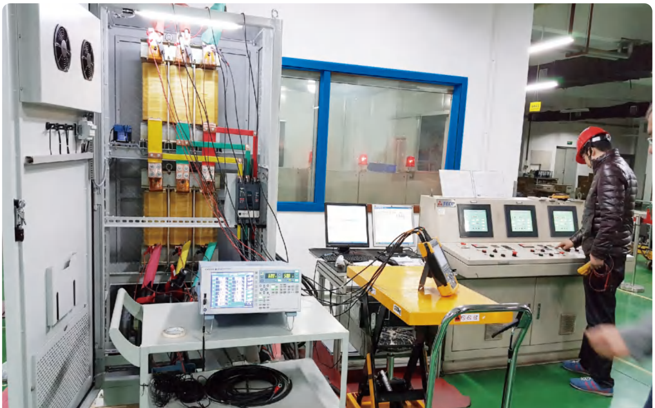
Passive harmonic filter performance testing
